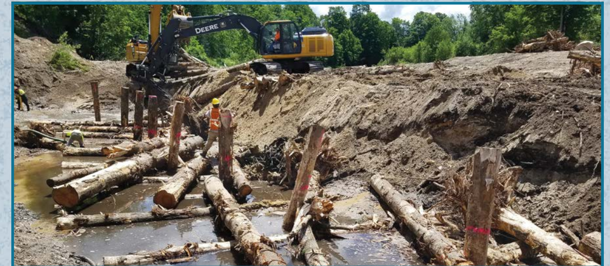
Logs and intact roots are recessed into streambanks and secured to the stream bottom to provide habitat and strengthen outside bends. (June 2017)
