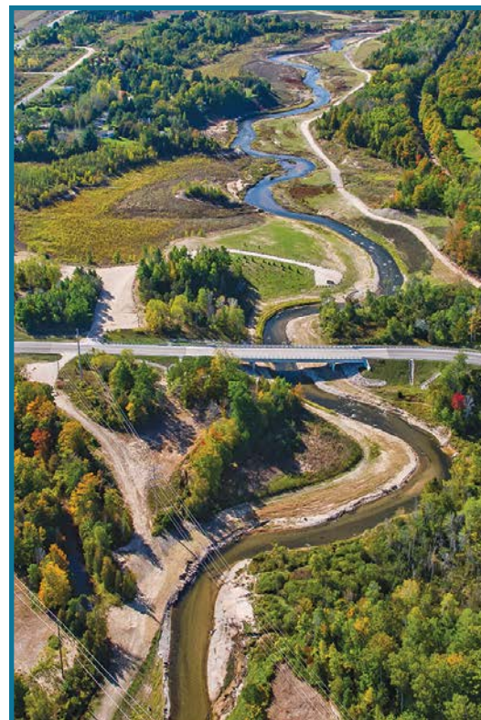
The river was returned to its original channel flowing under the new Robbins Bridge on Cass Rd. (Oct. 2019)
