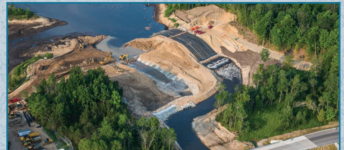
Gravity-fed siphons lowered the impoundment 21’ and an auxiliary spillway (left) drained the remaining water so the siphons could be removed and the river channel built in their place. (July 2017)
